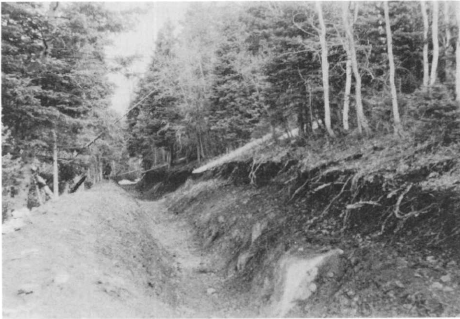
The Federal Work Progress Administration dug a ditch and syphon as part of the Payson City irrigation system. A small earth-fill dam was also constructed. (Manuscript Division, J. Willard Marriot Library, University of Utah)
