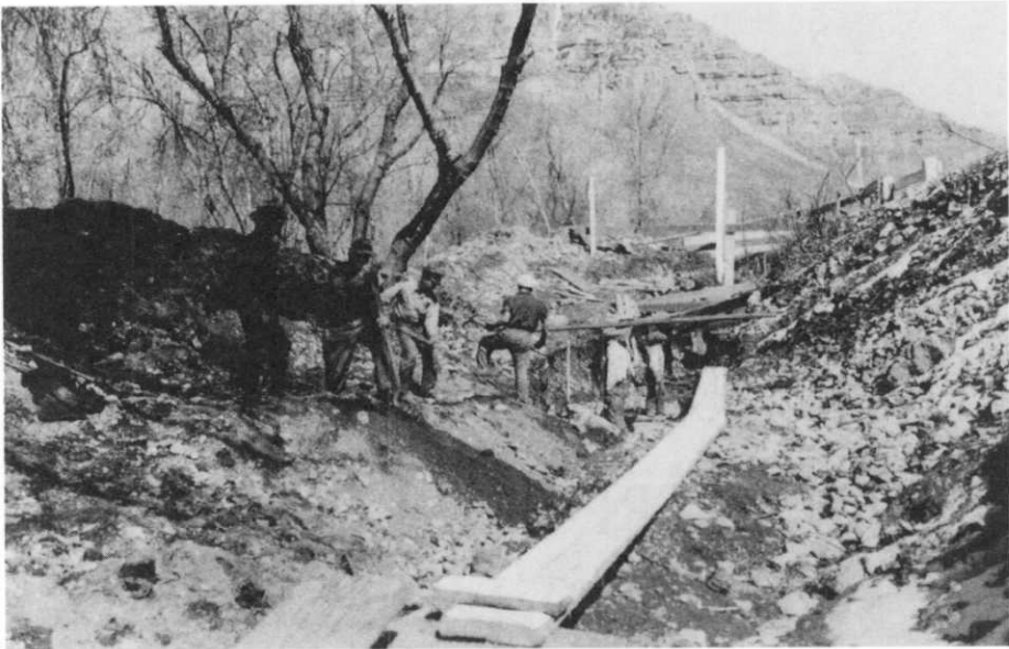
The Federal Work Progress Administration installed about seven thousand feet of twenty-four inch concrete culinary pipeline and built thirty-two hundred feet of retaining wall in Provo Canyon at a cost in excess of $100,000. (Manuscript Division, J. Willard Marriot Library, University of Utah)
