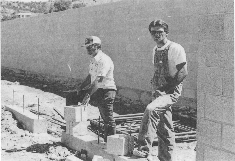
Construction of horse stalls at the Beaver Race Track in 1978. (Courtesy J.D. Osborn)
